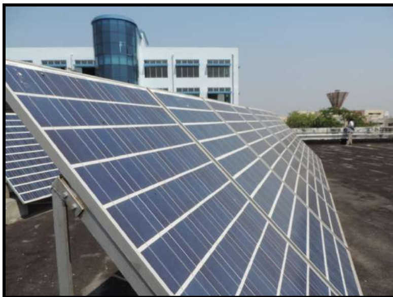
Photograph 2.3: Solar panels on the terrace
